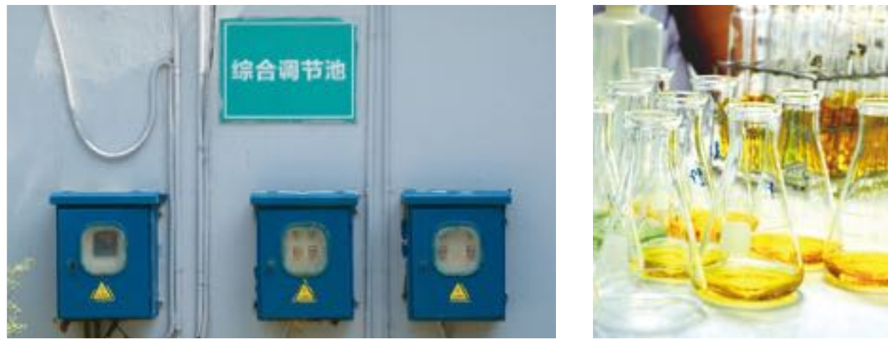
Sewage treatment system
